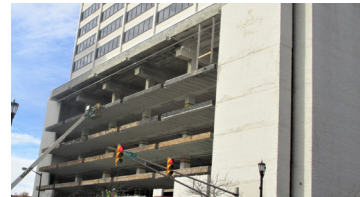
ALOFT HOTEL STRUCTURAL REHABILITATION AND RENOVATION SOUTH BEND, INDIANA PARKING STRUCTURE AND HOTEL SECTOR / COMPLETED 2016
