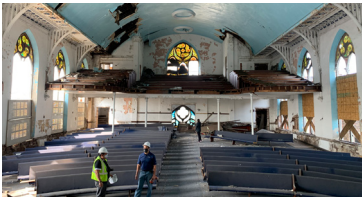
ST. STEPHENSON MISSIONARY BAPTIST CHURCH STRUCTURAL CONDITION ASSESSMENT FOR THE PRESERVATION OR DECONSTRUCTION CHICAGO, ILLINOIS RELIGIOUS SECTOR / DECONSTRUCTED 2021
