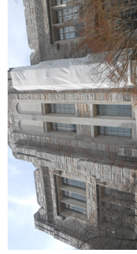
BUTLER UNIVERSITY JORDAN HALL STONE VENEER CONDITION EVALUATION INDIANAPOLIS, INDIANA CONSTRUCTION COST N/A YEAR COMPLETED 2013
