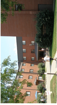
VINCENNES UNIVERSITY MULTIPLE ROOF CONDITION ASSESSMENTS VINCENNES, INDIANA CONSTRUCTION COST N/A YEAR COMPLETED 2007
