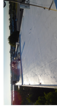
IVY TECH COMMUNITY COLLEGE FAIRBANKS BUILDING ROOF REPLACEMENT INDIANAPOLIS, INDIANA CONSTRUCTION COST $764,666 YEAR COMPLETED 2017
