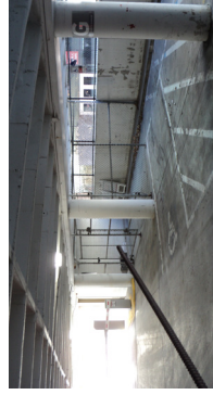
THE OHIO STATE UNIVERSITY NORTH UNION PARKING STRUCTURE RENOVATION COLUMBUS, OHIO CONSTRUCTION COST $2.6 million YEAR COMPLETED 2017
