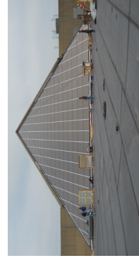
INDIANA UNIVERSITY FINE ARTS MUSEUM REROOF AND ATRIUM SKYLIGHT REPAIR BLOOMINGTON, INDIANA CONSTRUCTION COST $366,000/$585,000 YEAR COMPLETED 2008/2011
