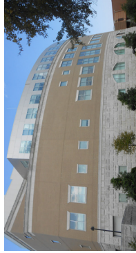
UNIVERSITY OF SOUTHERN INDIANA BUILDING ENVELOPE INVESTIGATIONS EVANSVILLE, INDIANA CONSTRUCTION COST N/A YEAR COMPLETED 2016
