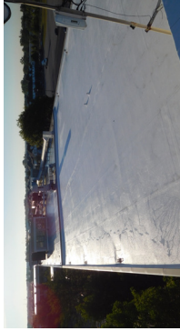
IVY TECH COMMUNITY COLLEGE FAIRBANKS BUILDING ROOF REPLACEMENT INDIANAPOLIS, INDIANA CONSTRUCTION COST $764,666 YEAR COMPLETED 2017
