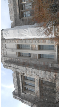
BUTLER UNIVERSITY JORDAN HALL STONE VENEER CONDITION EVALUATION INDIANAPOLIS, INDIANA CONSTRUCTION COST N/A YEAR COMPLETED 2013
